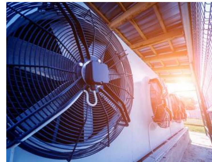
Heating, Ventilation, Air Conditioning and Refrigeration (HVACR)
